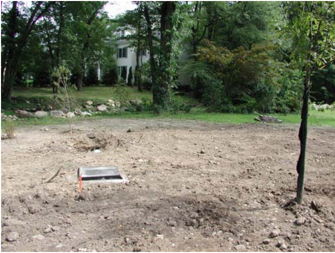
Partially completed drainage sans erosion controls, supervision or approval.
